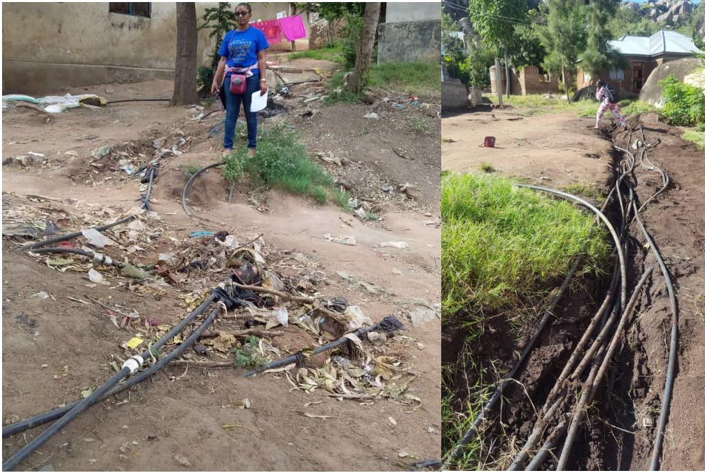
Figure 24: Picture showing spaghetti service lines in the study area extended for long distance from the mainline
